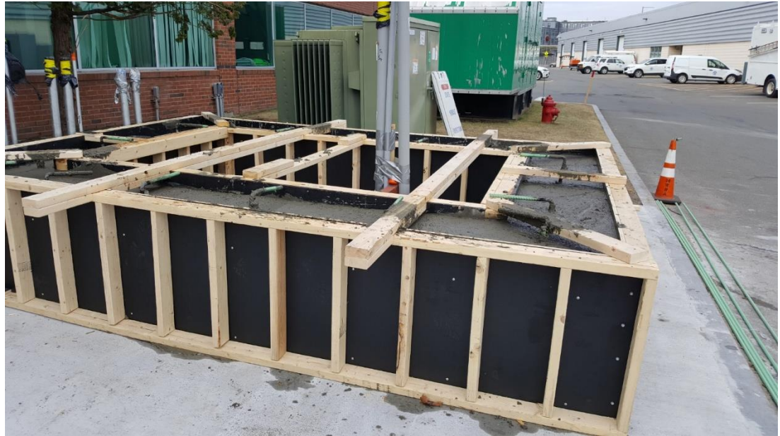
Chelsea Battery Storage Pad
